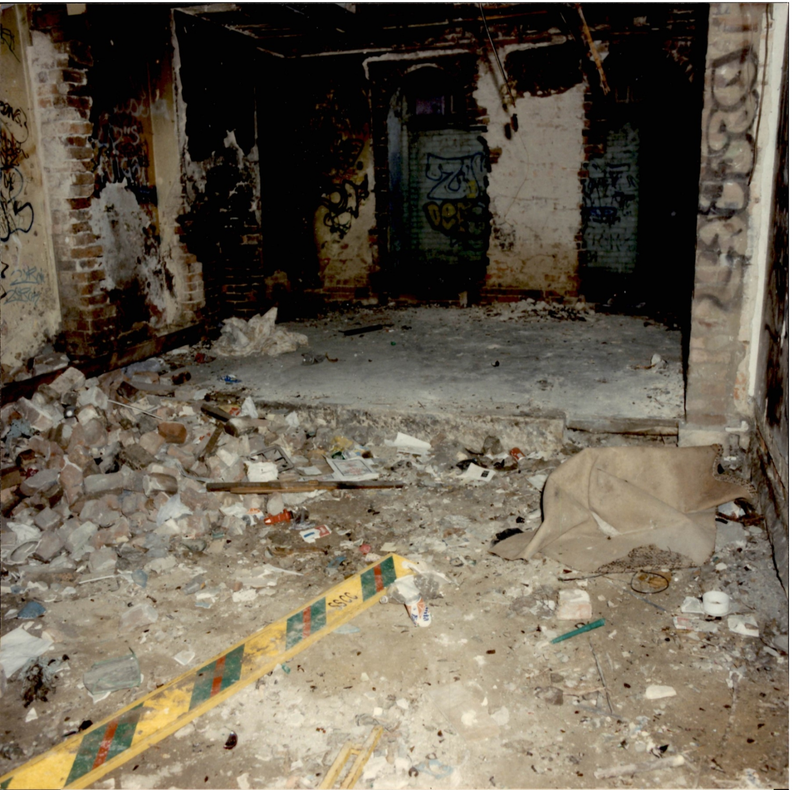
4. View of the ground floor in a westerly direction towards Everleigh Street.
